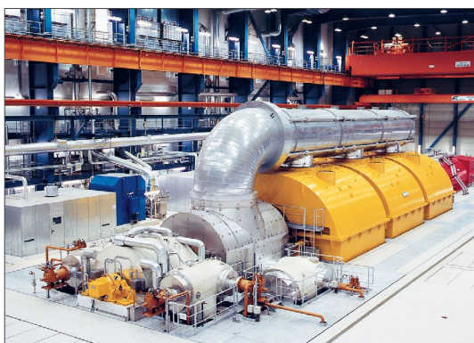
Typical production turbine used in large-scale powerplants. The project described called for each turbine to be secured individually.
