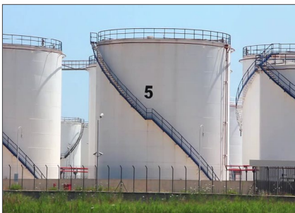
Oil storage tanks include a host of security measures, both physical and cyber. Each tank houses multiple sensors and controllers that control the environmental conditions inside the tank.
