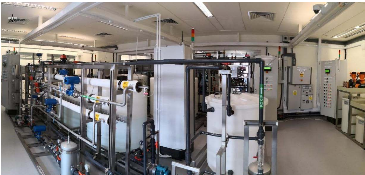
The SWaT Lab, simulating a real-life water treatment plant
